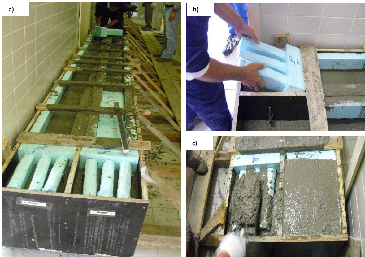
Figure 124 - First stage of the specimen's production: a) filling the formworks with concrete until it reaches the tension reinforcement level; b) insertion of the negatives at the supports; c) filling with concrete the support areas
