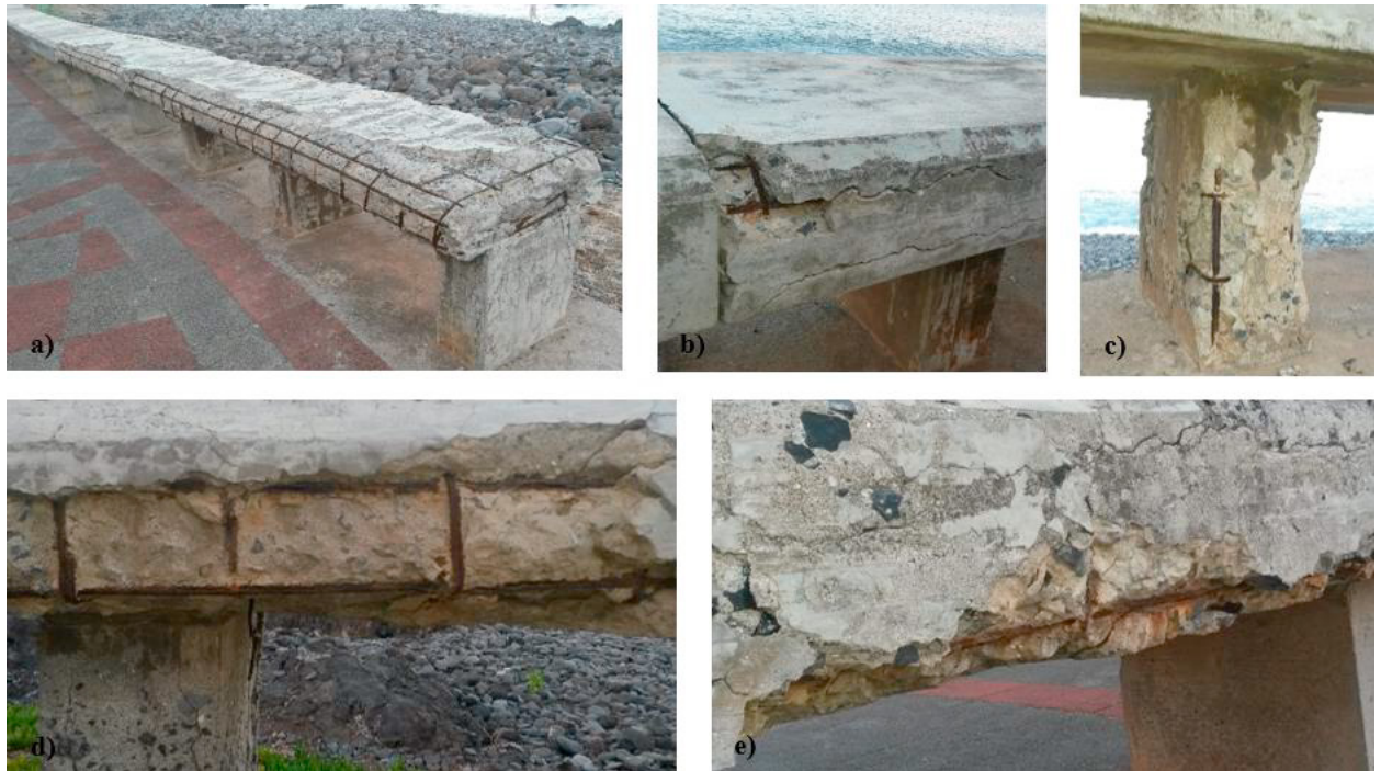
Figure 6. Fence / concrete bench: a) Element overview with delamination in the edges; b) Detail of cracking and spalling; c) Detail of a support with spalling on the edges; d) Detail of the concrete and the steel rebars disappeared; e) Detail of the aggregates dimension of the concrete.
