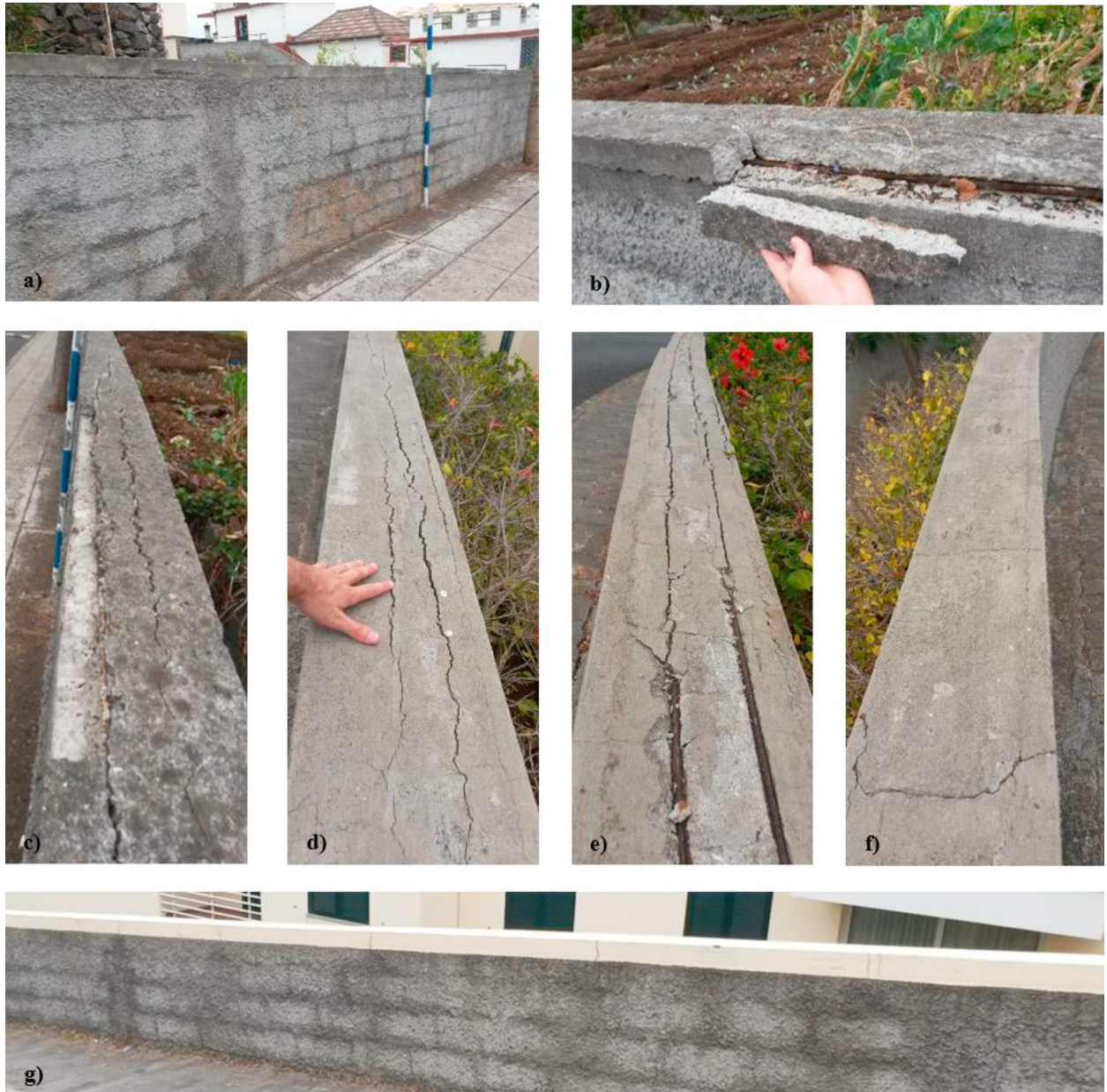
Figure 3. Concrete block wall with mortar at the top: a) Element overview; b) Detail of the spalling of edges; c) Advanced cracking and spalling of edges; d) Cracking part; e) Cracking over corroded rebar; f) Detail of the transversal cracking not avoided g) Alternative concrete block wall having transversal cracking but no corrosion and longitudinal cracking.
