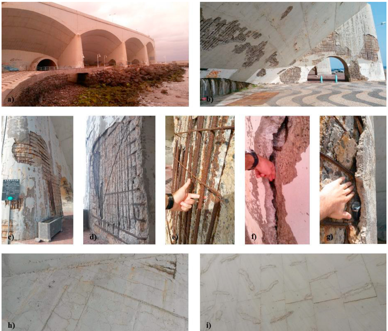
Figure 5. Concrete buttress arch: a) Construction overview; b) Generalized spalling; c) Buttress; d) Advanced spalling with disappearing of the rebars; e) Disassemble of the steel rebars; f), g) Gaps between the cover and buttress core; h) Overall cracking; i) Repairing points.
