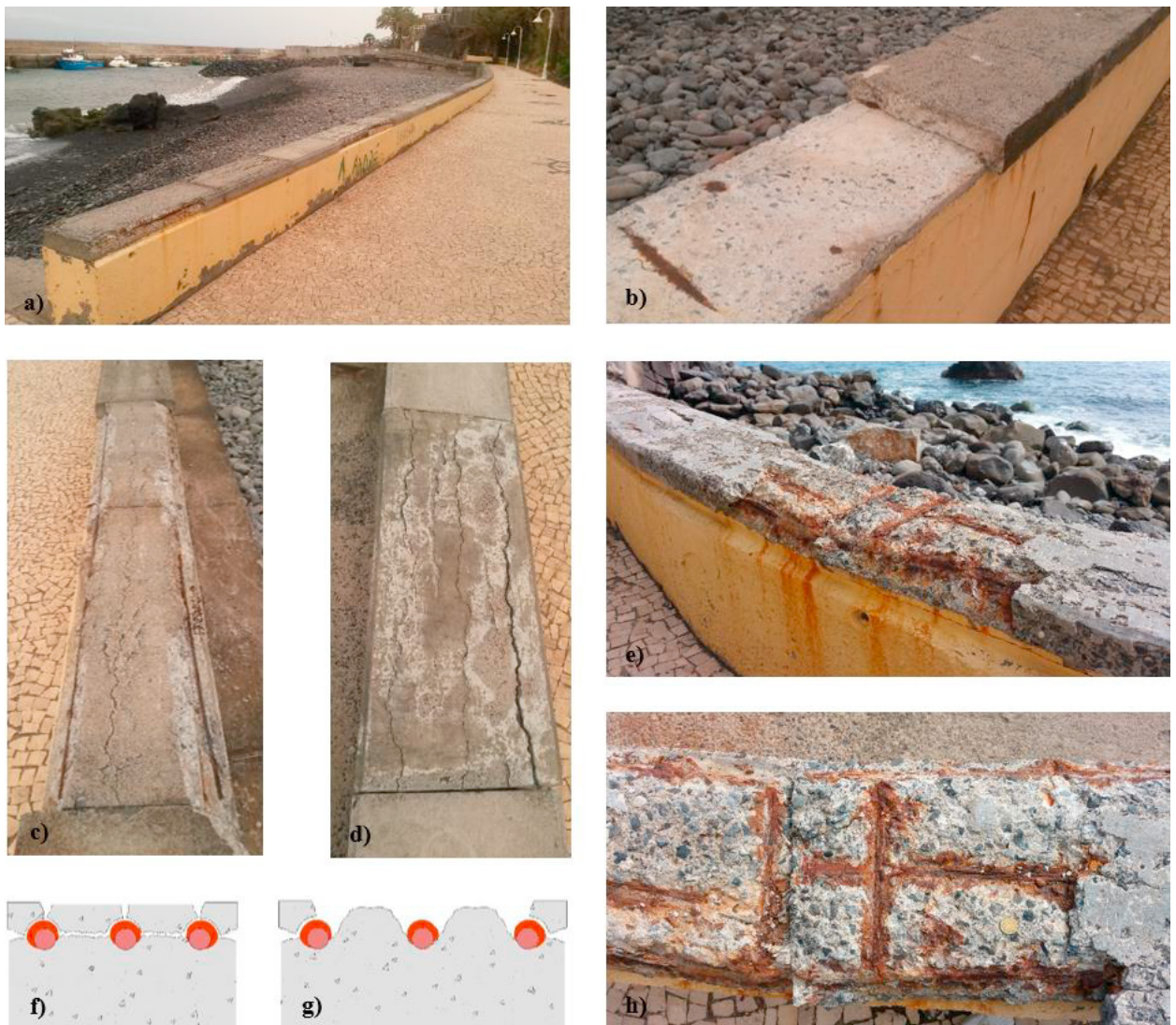
Figure 2. Fence / sitting concrete wall: a) Element overview; b) Construction with two distinct elements; c) Spalling of edges; d) Advanced cracking of the prefabricated element (cover); e) Full corrosion and delamination of the cover (not prefabricated); f, g) Scheme of the reinforcement corrosion and consequent cracking and delamination; h) Detail of the deterioration of the cover in the no prefabricated element.
