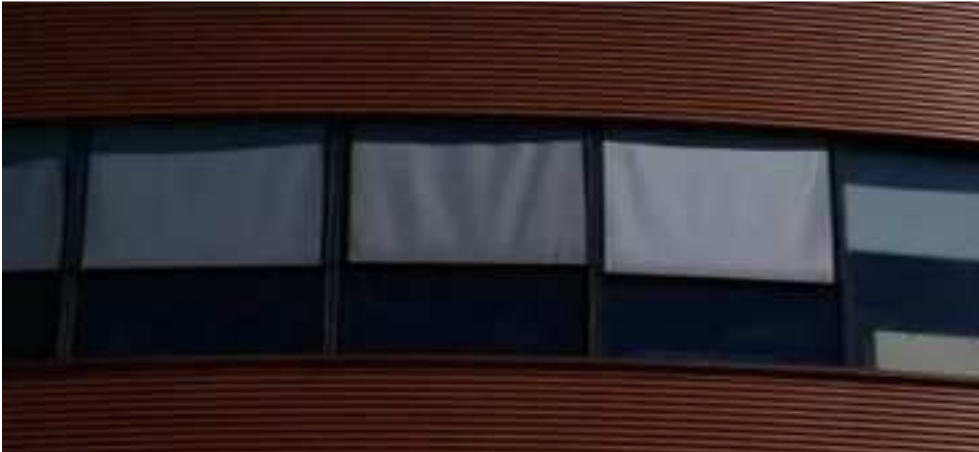
Picture 5.8: Lighting control with interior blinds. Source: rtvslo
